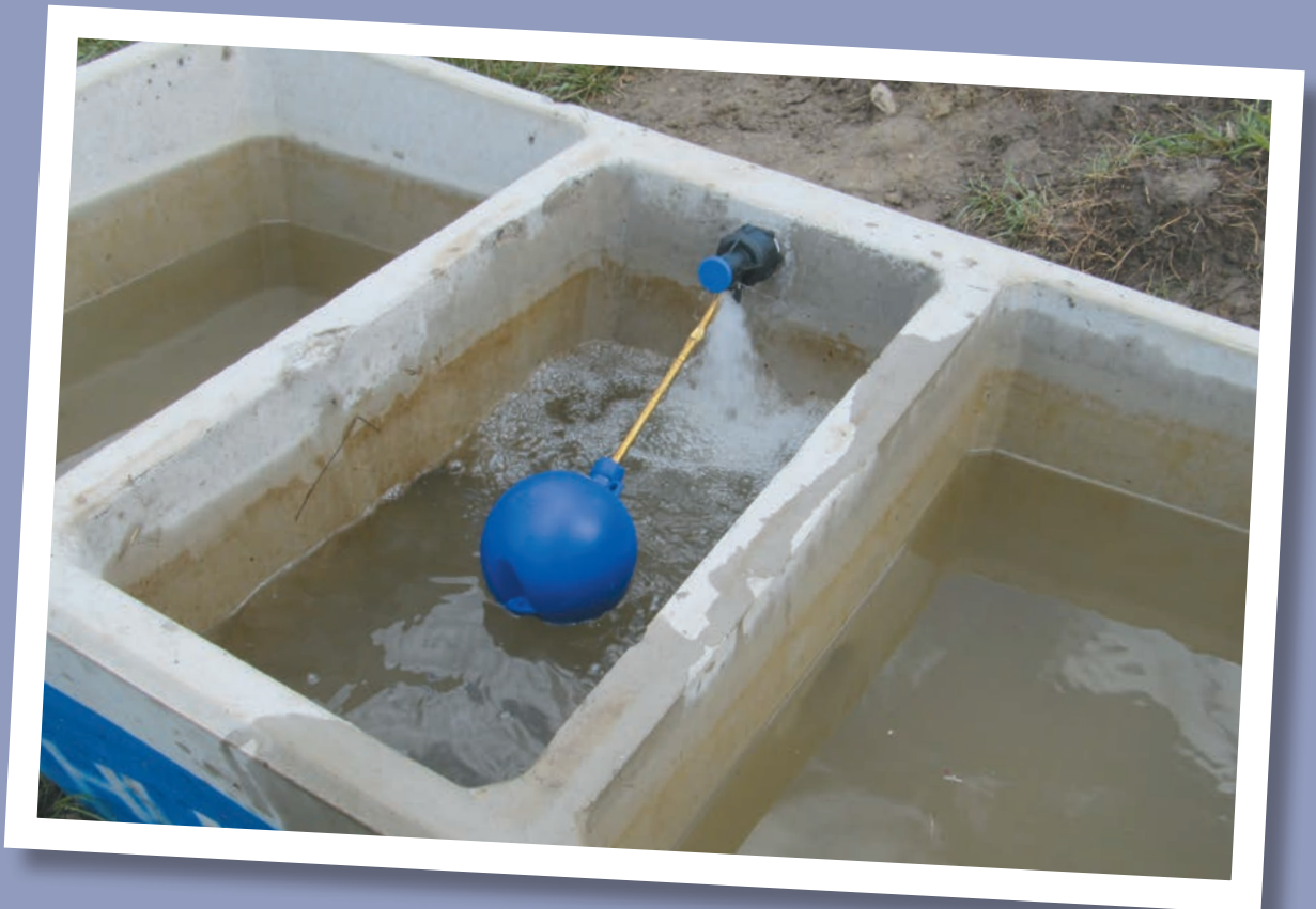
Hansen Fastflo Valve (HFFSV) in use
