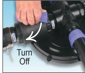
Step 2. Proceed to turn all the Pod Sprinkler Lines Valves off at the Pod Hydrants.
