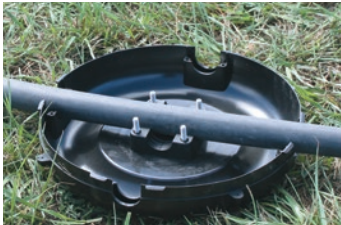
Lay pipe over Skid Base and secure in position with Cross Tee Anchor.
