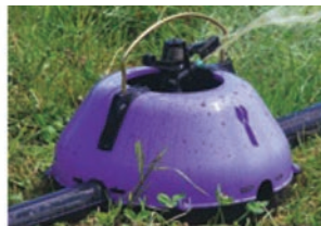
Irripod Lilac Effluent System
