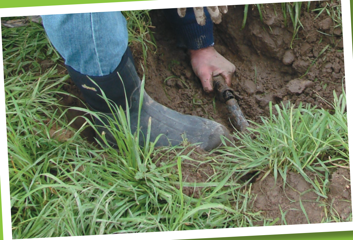
Hansen Reducing Straight Coupling (HRS) in use
